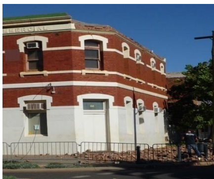
Above: a pile of rubble is all that remains of the parapet from the top of this building in Burt Street, Boulder.
